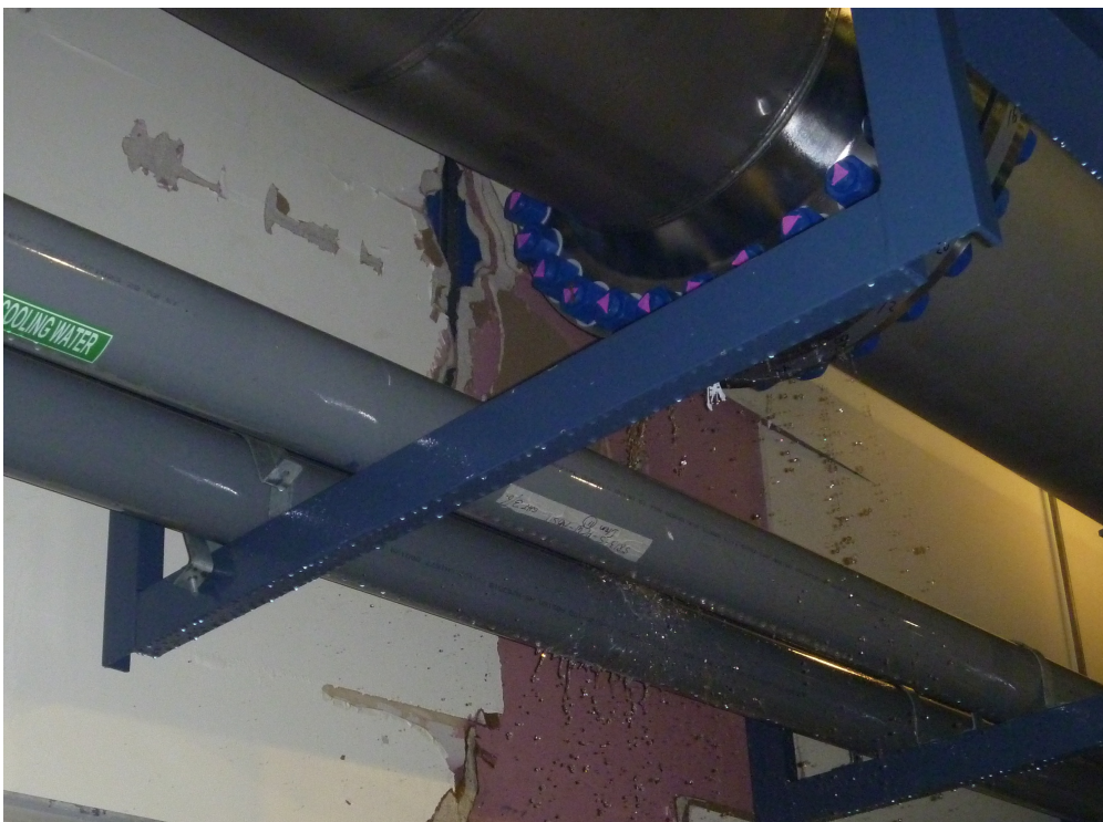
Figure 1: Damage to building due to high pressure flange failure
