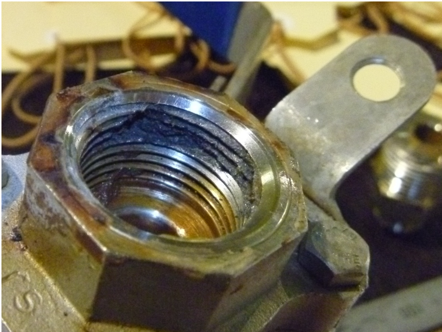
Figure 2: Example of corrosion of threaded fittings encountered in RO seawater desalination service
